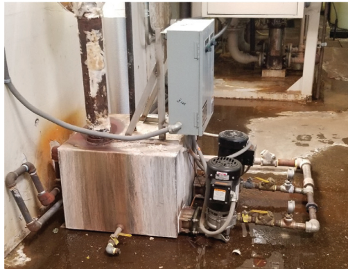
FIGURE 2. This pump station exhibits severe spillage, creating a potential safety hazard and source of problems
