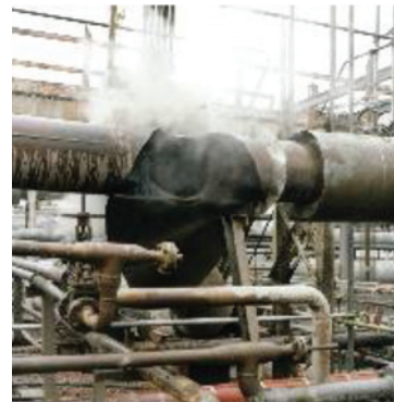
Figure 1. Failure of a steam distribution line at a combined refinery and petrochemical complex. [2]
