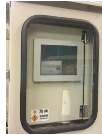
Control panel for outdoor specifications
