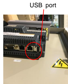
Figure: Inside the control panel
