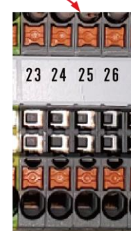
Operation Alarm output
