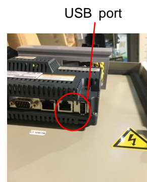
Figure: Inside the control panel
