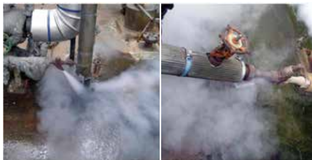
▲ Figure 2. Opened bleeds on steam tracing lines are a sign of poor heat transfer, and may be indicative of faulty steam traps.
