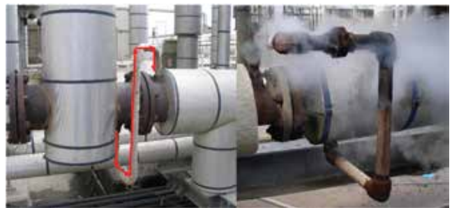
▲ Figure 13. If standard traps are used on jacketed piping with S-loop connectors (red), steam bleeds (like the one shown on the right) likely indicate heating issues.
