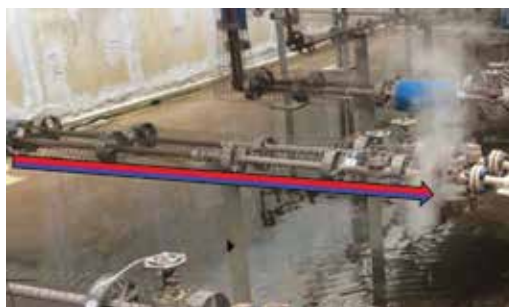
▲ Figure 16. Long horizontal piping runs to the traps created steam locking issues, which were resolved by adding a steam trap with an internal bypass.
