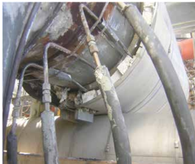
▲ Figure 1. This pipe has multiple steam tracing lines installed to obtain high heat transfer.
