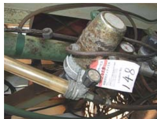
Leakage from the regulator
