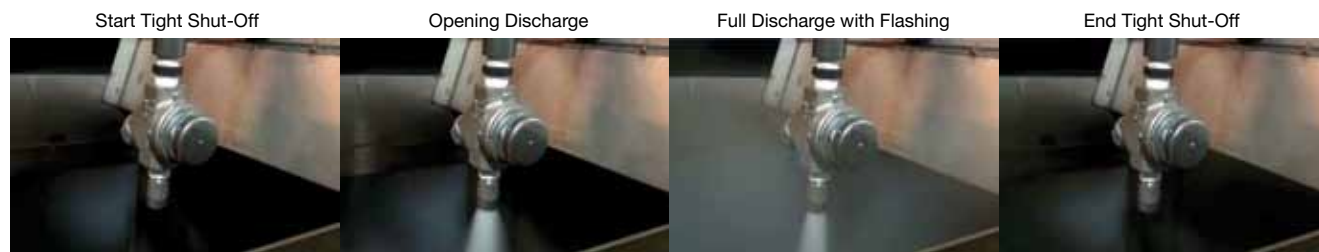
▼ Figure 3. To look for condensate drainage, a trap should be taken through the four stages of operation (as shown in these images for a vertical trap with 580-psig steam).
