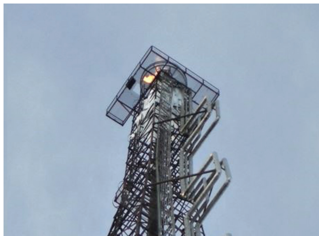
▲ Figure 3. Ice formation at the top of a flare can be evidence of excessive condensate in the steam supply; it creates a safety hazard that should be mitigated.
