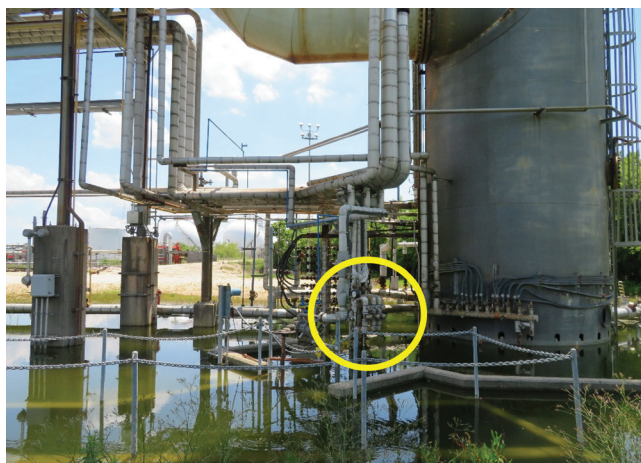
▲ Figure 11. Improper steam trapping is at least part of the cause for the pond that formed beneath this flare.
