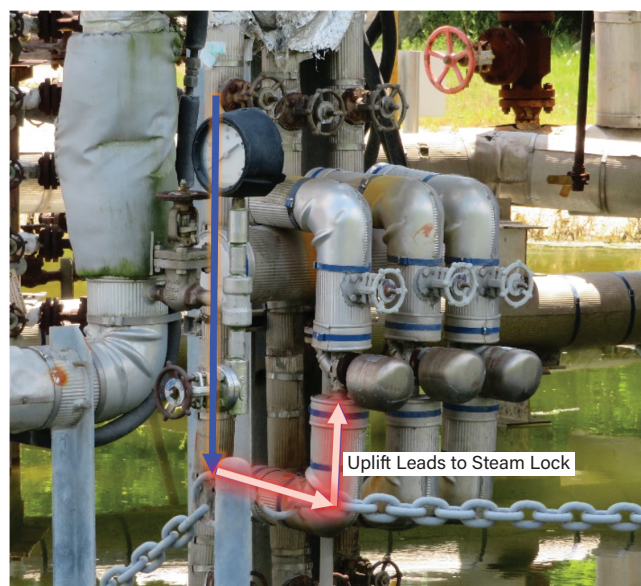
▲ Figure 12. Generally, trying to uplift condensate to a steam trap will create a steam lock; this type of improper installation should be avoided.
