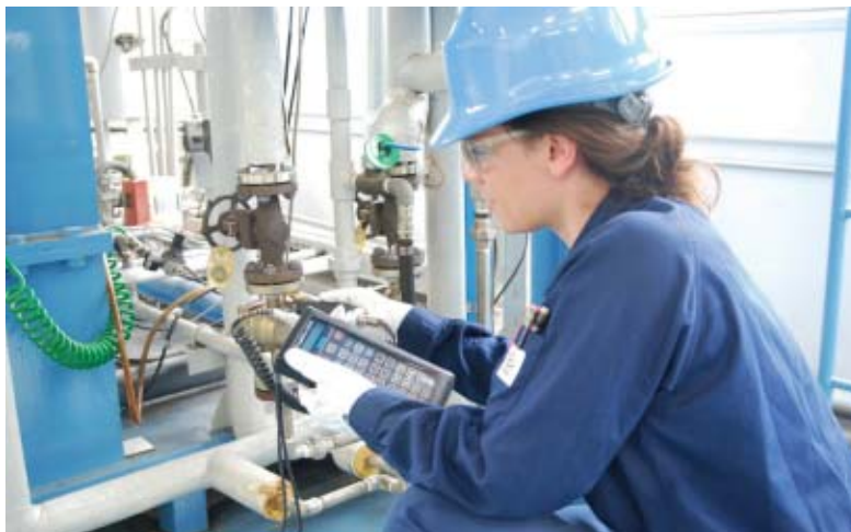
FIGURE 3. Accurate and regularly sustained diagnosis of steam traps’ operating conditions is essential to determining the population’s current health (state of the population). Once failures are identified, the information is valuable for allocating resources to restore all condensate discharge locations to an “as designed” operating condition for safety and reliable performance
