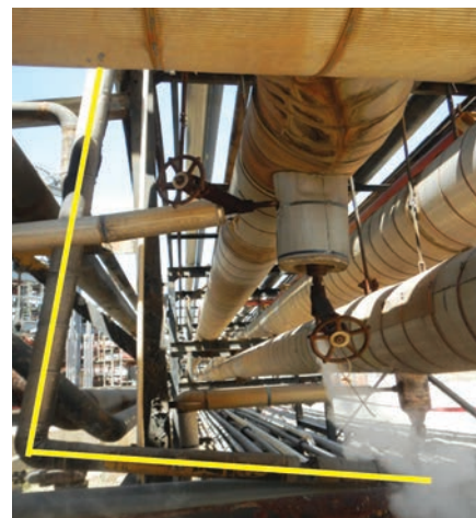
FIG. 12. This 24-in., 220-psig superheated steam line had a 400-ft section moved 7 ft by slug hammer.
