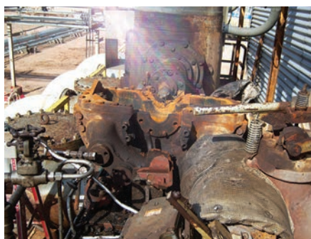
FIG. 8. The potential damage caused by slug-induced water hammer should not be underestimated.
