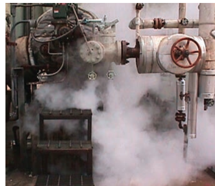
FIG. 11. Fog zones can create visual hazards and still be ineffective to mitigate turbine damage.
