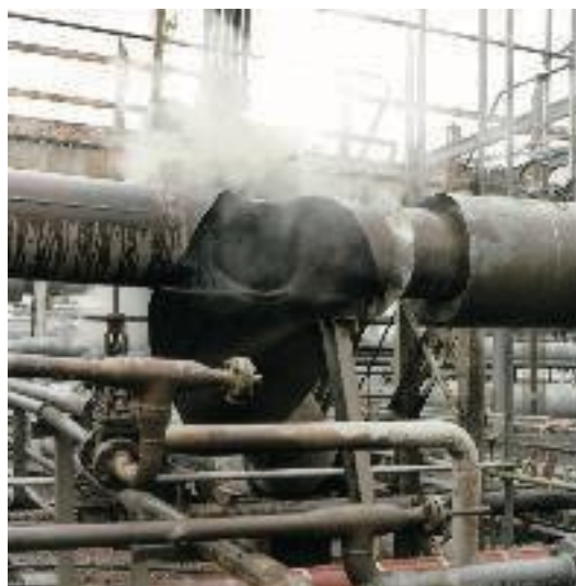
▲ Fig. 12. Significant blow-out of a steam pipe due to a water hammer event (BP Grangemouth, 2000).
