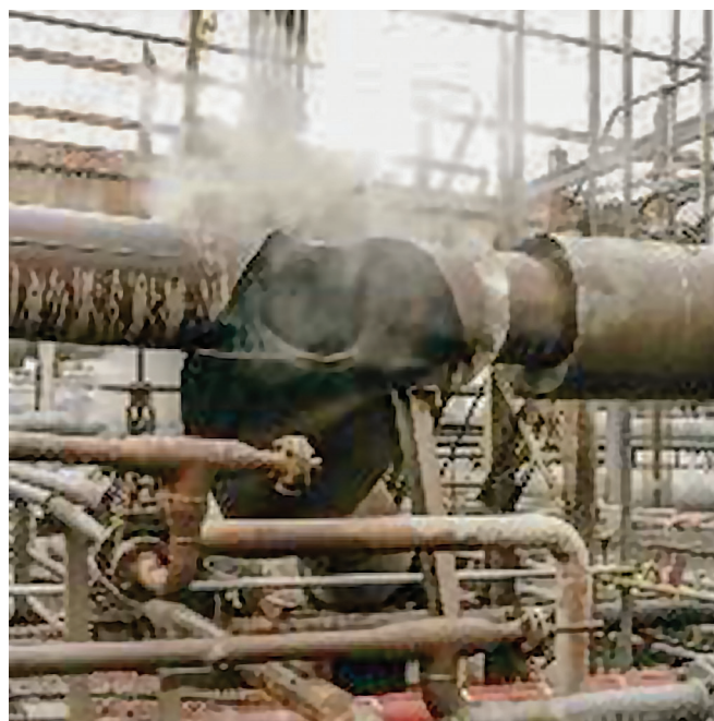
FIG. 2. Failure of a steam pipe joint due to water hammer.
