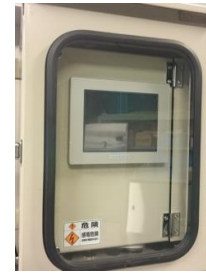
Control panel for outdoor specifications
