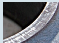
Wall thinning caused by steam leakage from eroded valve trim.
