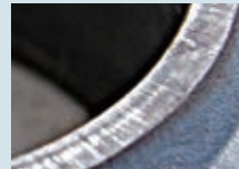
Wall thinning caused by steam leakage from eroded valve trim.
